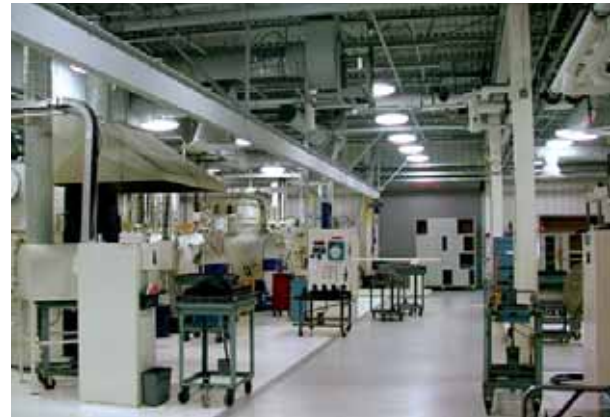
Heat treatment plant completed in the fall of 2005.
